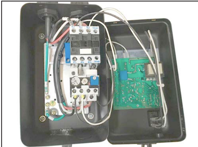
Figure 81. Control box wired for 220V operation.
