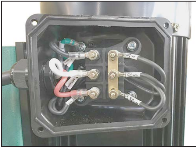
Figure 80. Motor wired for 220V operation.
