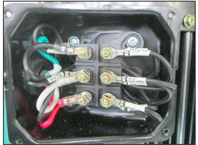
Figure 83. Motor wired for 440V operation.
