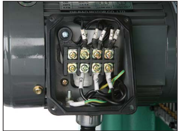
Figure 75. Vertical motor wiring.
