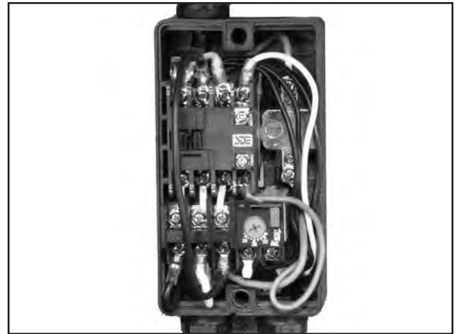
Figure 15. 220V magnetic switch
